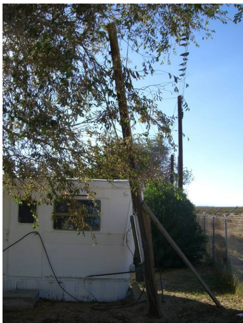
Leaning/Unstable Power Pole
