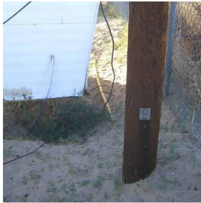
Exposed Natural Gas Line
