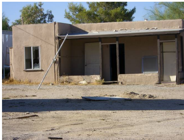
Common Area Building with Broken Windows and Doors
