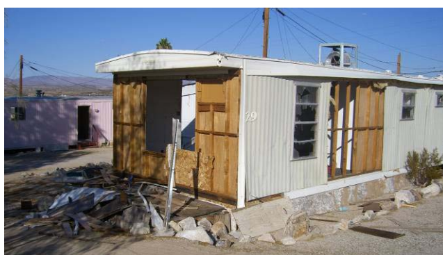
Mobilehome under Reconstruction with Glass and Other Dangerous Materials Exposed for Children
