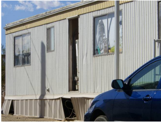
Missing Hot Water Heater Door and Damaged Skirt with Sharp Metal Edges
