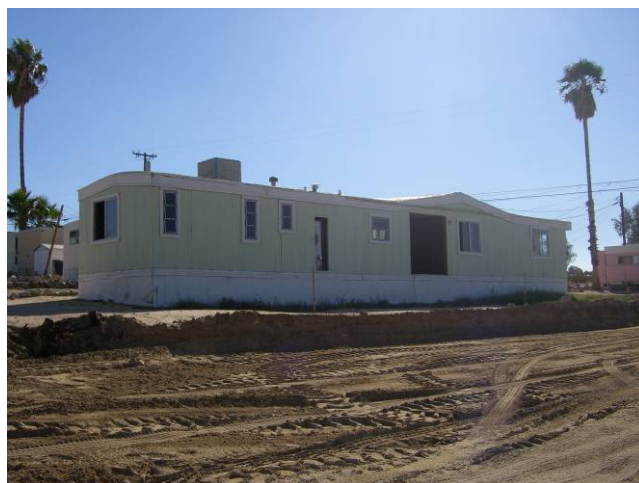
Mobilehomes without Windows and Doors along New Roadway Adjacent to New Subdivision
